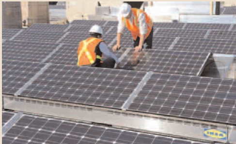
Ikea has erected a large solar panel installation on the rooftop of its Etobicoke store. — Photo by Colin McConnell / Toronto Star
